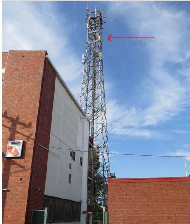
Image showing existing Tower with 1.2m dish identified
