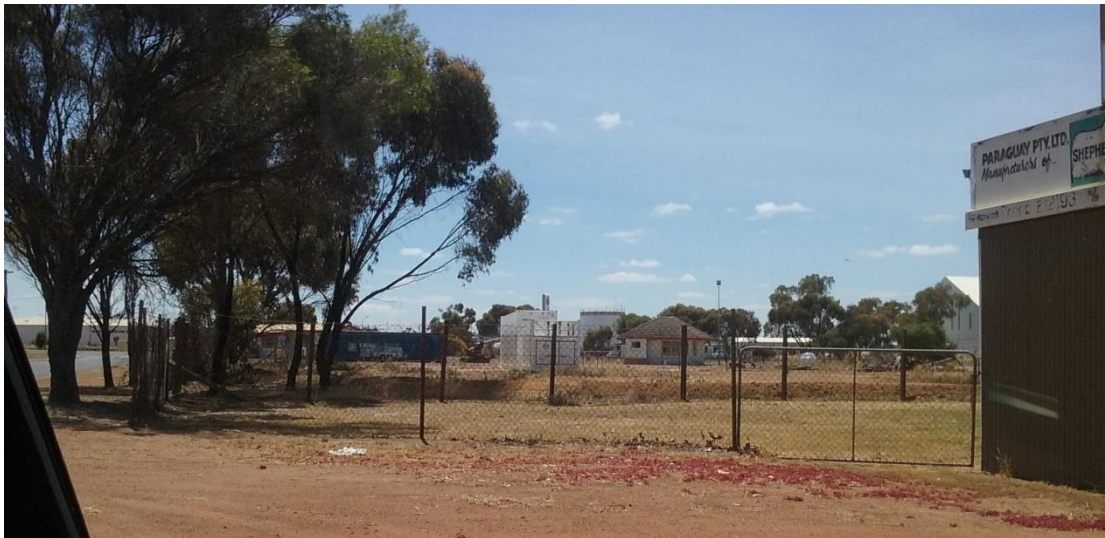
Rear/northeast view of development site during preliminary construction with Bay Street on left, new above ground diesel storage tank and former, decommissioned building [December 2016].
